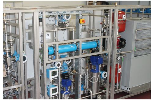
Reverse osmosis for seawater desalination
